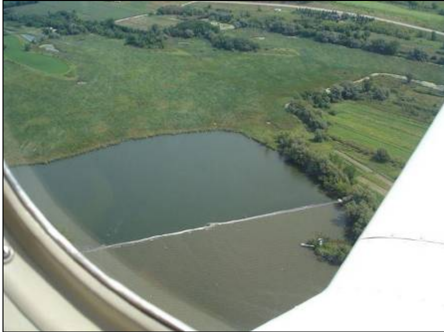
Figure 13. "Aerial photograph of Geotube breakwater structure and sediment berm on Lake Sinissippi, showing improved water clarity within contained 24-acre embayment. Installation completed in May 2006. Photograph taken August 2006."
