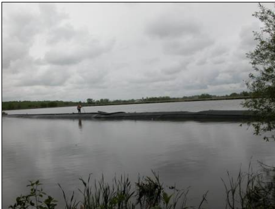
Figure 14. Geotube geotextile containment tubes, 760 feet long. Note: These tubes are functioning as breakwater across opening to 24-acre embayment to stabilize shoreline and existing wetlands, reduce the flow of sediment to lake from creek that empties into the back bay, provide mechanism to reestablish aquatic macrophyte community, improve habitat for waterfowl, and enhance hunting and other recreational activities. Lake Sinissippi at Wildcat Road, May 2006.
