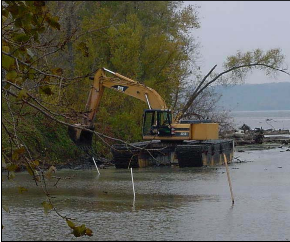
Figure 8: Floating Excavator As stated previously, floating excavators are ideal for those hard to reach places and are highly mobile. However, they are not as efficient as the other types of machines.
