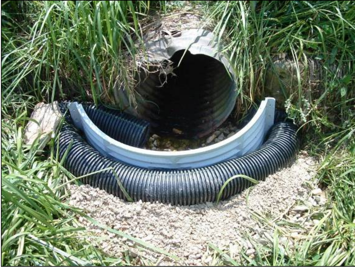
Figure 11. Galvanized steel collar, gravel and drain tile on Lake Drive road culvert that drains into Lake Sinissippi. The culvert collar traps sediment flowing in road ditches, while allowing clear water to pass into the culvert and flow to the lake. LSID worked with the local township to install several sediment retention structures on road culverts in 2006.
