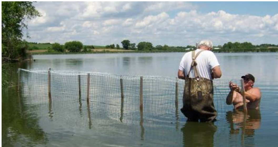
Figure 17: Protective screened enclosure being installed in the embayment behind the Geotube breakwater. The water depth is about 2 feet. A screen is being attached on the top of the enclosure to prevent access to Canada geese and other herbivorous birds. American lotus seeds and rootstock of water lily species were planted in the sediment within the enclosure. Lake Sinissippi - 2009
