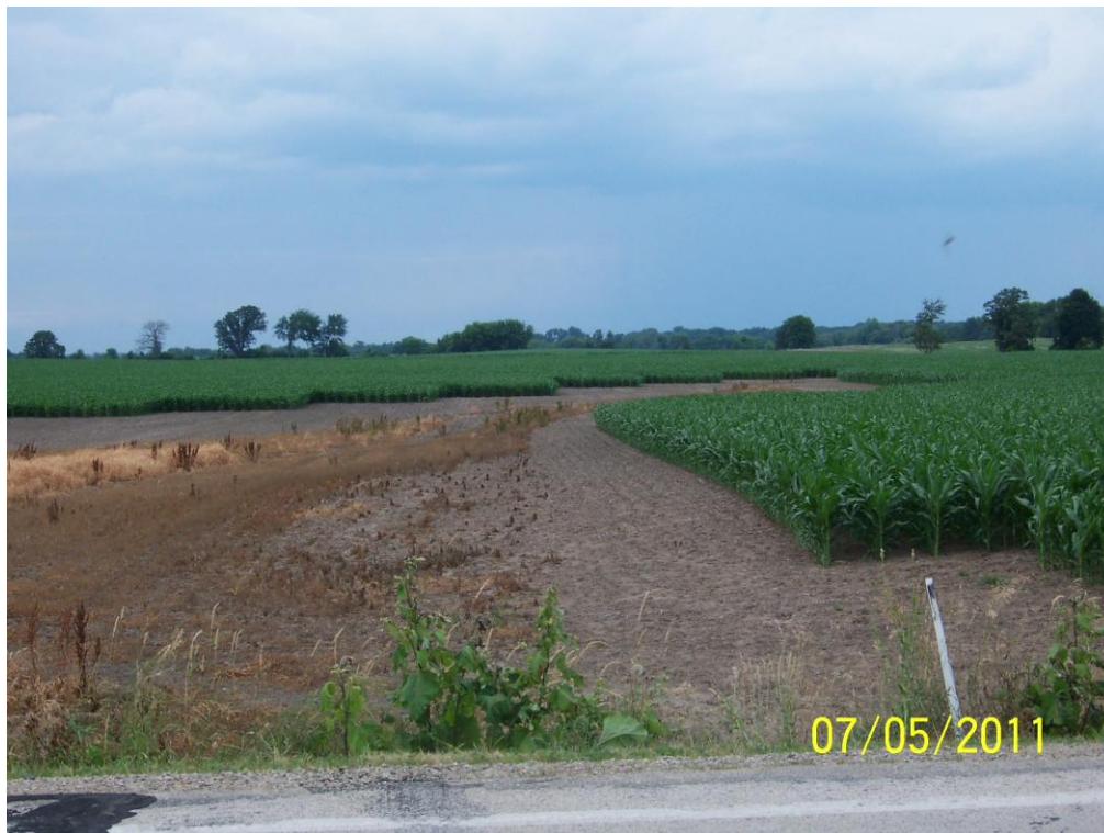
Figure 8. Looking north from culvert at Highway B showing the drainage way with an herbicide-treated zone near the centerline of the drainage way and bare, exposed soil with no cover vegetation on either side of the centerline.
