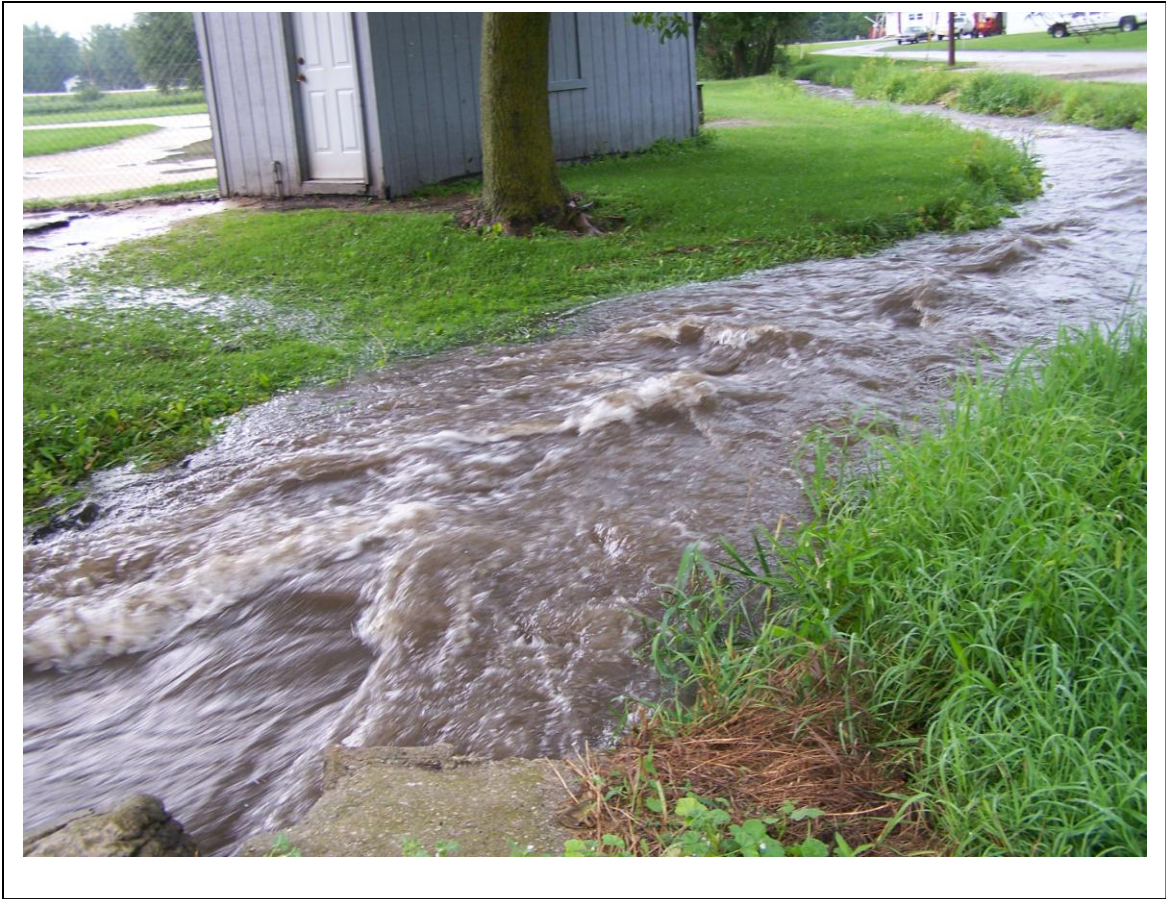
Figure 10. Photograph taken July 22, 2010 of Spring Brook flowing from the culvert at Fireman's Park, Burnett, during a rain event. In the region of turbulence just downstream of the culvert, the creek has overtopped the north bank. A representative of the Burnett Sanitary District testified at the drainage board public hearing on July 13, 2010 and expressed concern about the increased quantity of surface water flowing to the community if the proposed drainage district is established.
