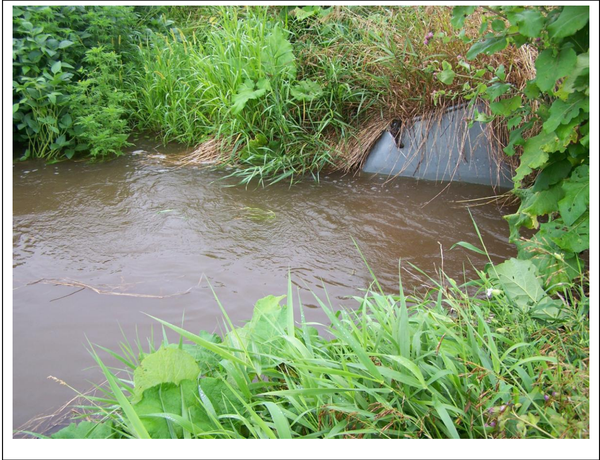
Figure 5. Culvert underneath Highway B, carrying drain water from the Dodge County Antique Power Club north to the Meylink soybean field. The culvert is 42 inches in diameter with a cross-sectional area of 9.62 ft 2 . At the time of measurement the water flow through the culvert was estimated at 20 ft 3 /s, equivalent to more than 500,000 gallons per hour. Photograph taken July 23, 2010.
