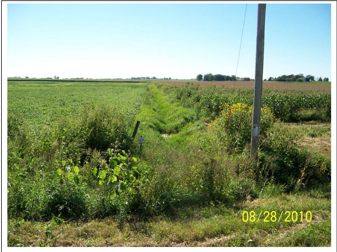
Figure 2. Existing field ditch at Road I culvert looking west. Agricultural field runoff from lands to the west, including those of the dairy livestock operation on Butternut Road, flows east in the drain ditch, through the culvert and then to the Dodge County Antique Power Club. This ditch is to become part of the district drain for the proposed Drainage District #88. The ditch appears to be in violation of state requirements given in §§ ATCP 48.24 and 48.30 that establish minimum 20-ft wide vegetative corridors on each side of a district drain, prohibit row cropping within ditch corridors and mandate erosion control measures to buffer against land uses that may adversely affect water quality in the ditch.
