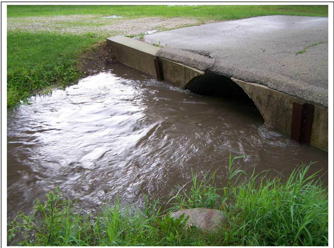
Figure 9. Photograph taken July 22, 2010 of Spring Brook flowing through a 6 x 4-ft culvert at Fireman’s Park, Burnett, during a rain event. The water flow of the creek is within 10 inches of over-topping the culvert. On either side of the culvert and bolted to the concrete structure are metal channels for stop logs. The stoplog dam is designed to adjust water level and reduce flow downstream to the community. However, during high-water conditions, such as existed during this rain event, the dam is ineffective in controlling flow and flooding occurs, as is shown in Figure 10.
